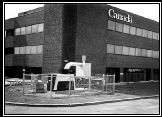
Microturbine unit providing 75 kW of electrical power as well as heat to a Health Canada building in Toronto (photo courtesy of Mercury Electric Corporation).
