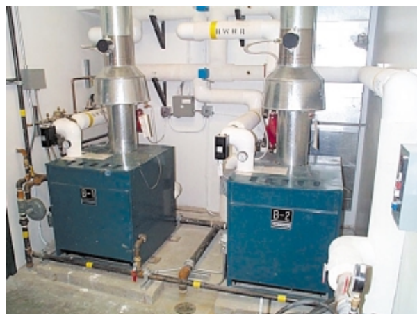
Figure 2 – Vent Damper Installation on Boilers
