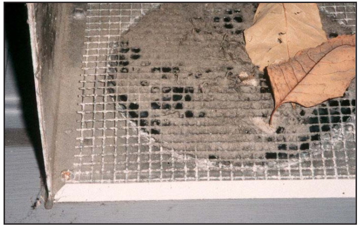
Figure 1: Blocked HRV intake
