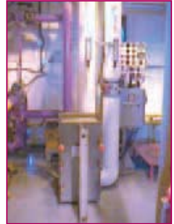
Main jacket water heat exchanger
