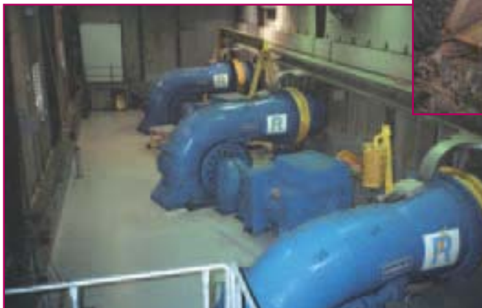
Black River – Penstock
