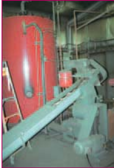
Wood Heating Boiler
