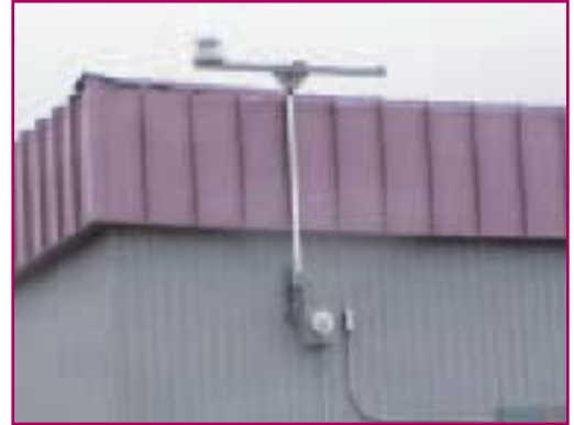
Part of the Nunatta Campus PV array system
