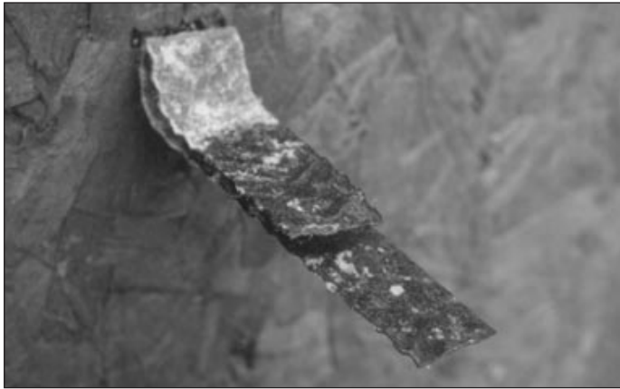
Figure 2. A galvanized, corrugated strip tie corroded on the part of the tie that was embedded within the mortar joint
