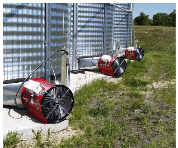
Aeration units - fans used to reduce grain moisture or temperature
