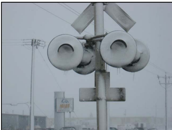
Photo 2. South signal, northward-facing lights
