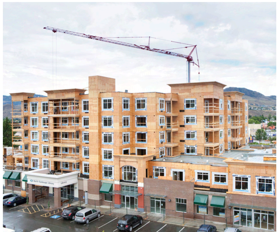
Five-storey wood-frame construction in Library Square in Kamloops, BC. Photo credit: Stephanie Tracey @ Photography West c/o WoodWORKS! BC
