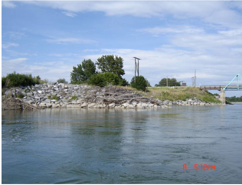
Figure 15. South bank of the Oldman River, immediately east of the Highway 811 bridge (in background), east side of the town of Fort MacLeod (facing southwest). Note manmade mesh bank armoring, likely to protect the bank from natural erosion forces. The spring and seep habitat required by S. bertae is so small that such anthropogenic disturbances could completely destroy the habitat. (Photo courtesy of Jennie Knopp.)
