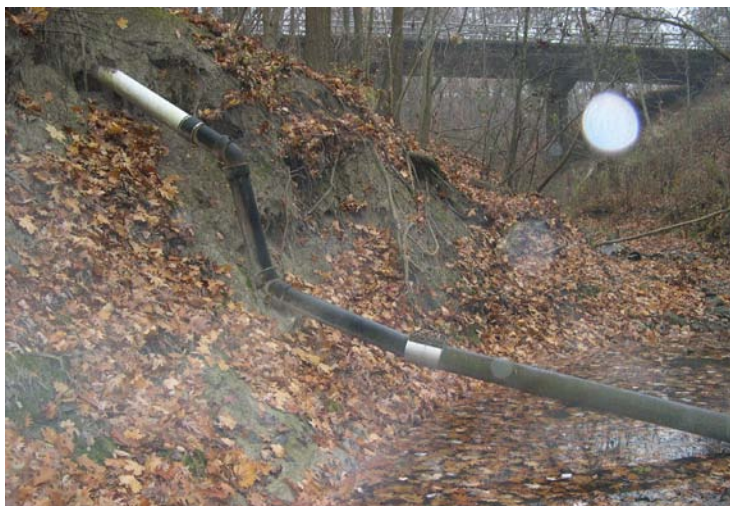
Figure 9. Recent repairs to an undercut, leaking sewer line at a stream crossing in Lake County, Illinois Photo by: Michael Adams, 2007
