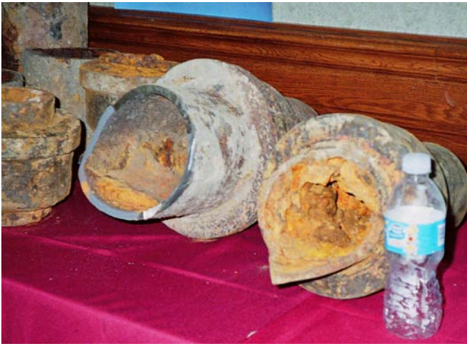
Figure 6. Examples of Windsor, Ontario's, rusty pipes with hardened scale corrosion. An eight-inch water main will become a two-inch main after about 50 years due to scale/precipitate build-up; an obvious problem for fire suppression in older municipalities. (Liquid Assets, 2008). Photo by: D.W. Alley, 2007
