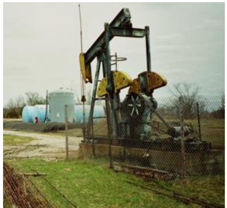
Figure 7. Brine well and storage tanks with secondary containment, Kent Co., Ontario Photo By: D.W. Alley, 2007
