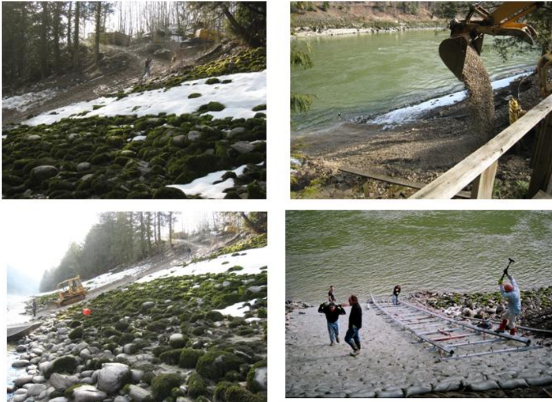
Photo 1. Right-bank modifications performed at the Qualark Creek hydroacoustic site on the Fraser River. The top left shows the removal of the existing surface layer and the top right shows the addition of the 10 cm crushed rock. The bottom left shows the levelling of the crushed rock and the bottom right shows the installation of the sandbag ramp and track system for the fish deflection weir.
