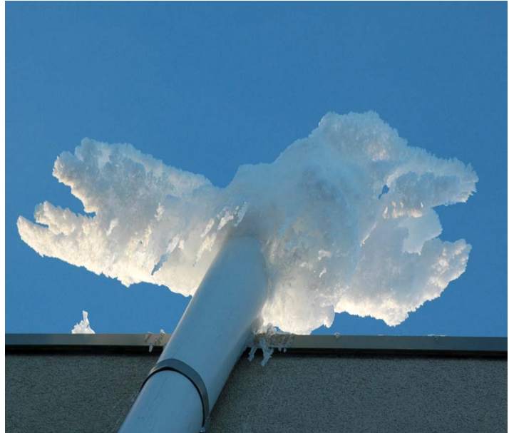
(radon vent, rain cap, ice sculpture photo credit Harry Johnson)
