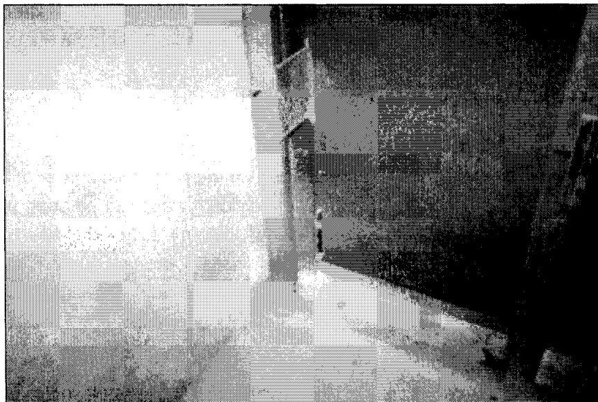
Figure 2.9: Hole Left Unsealed When Brick Tie Relocated
