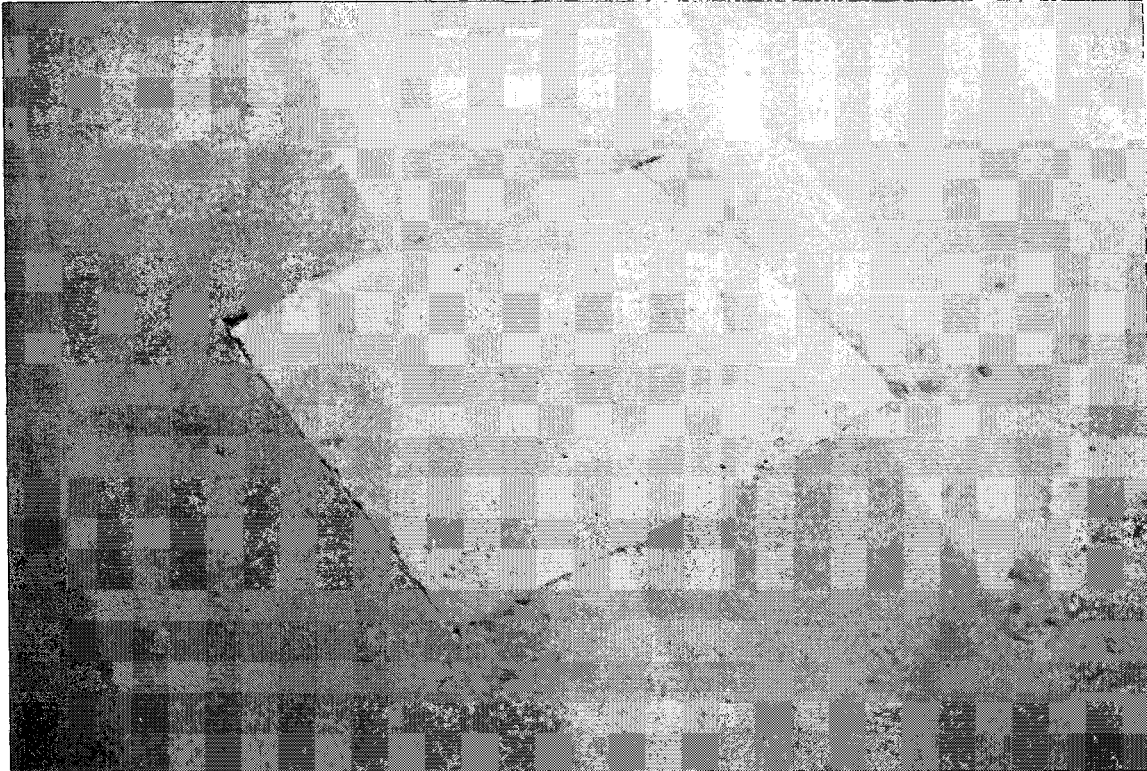
Photograph 1. Patching of shotblasted deck , level P2 at Ottawa City Hall, with an epoxy patching material.
