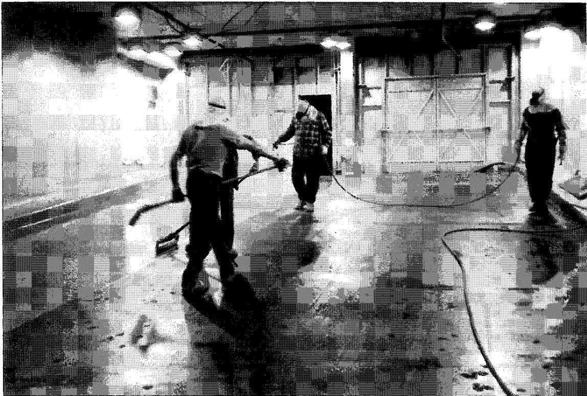
Photograph 6. Application of PDM3 by spray and back rolling at Ottawa City Hall.
