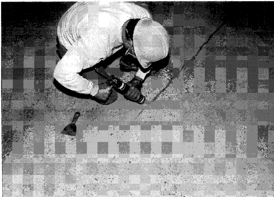
Photograph 2. Filling of routed crack with urethane joint sealant, level P2 at Ottawa City Hall.
