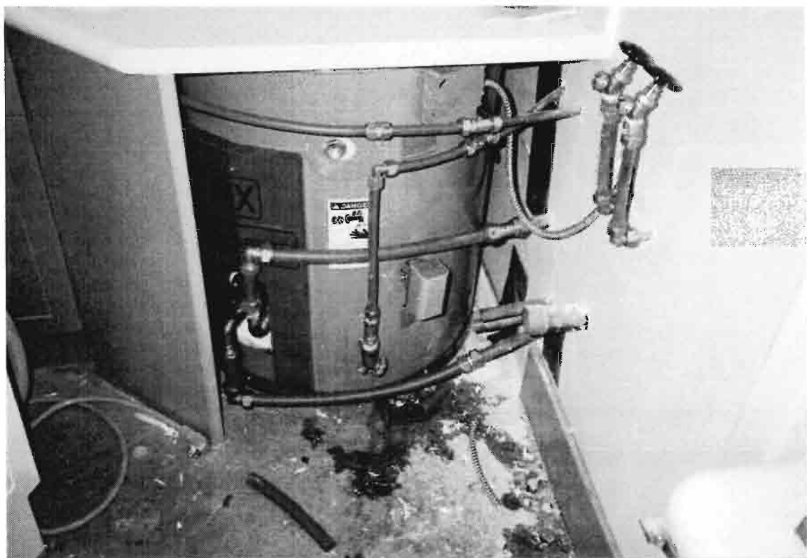
PHOTO 1-14 POTABLE HOT WATER TANK
