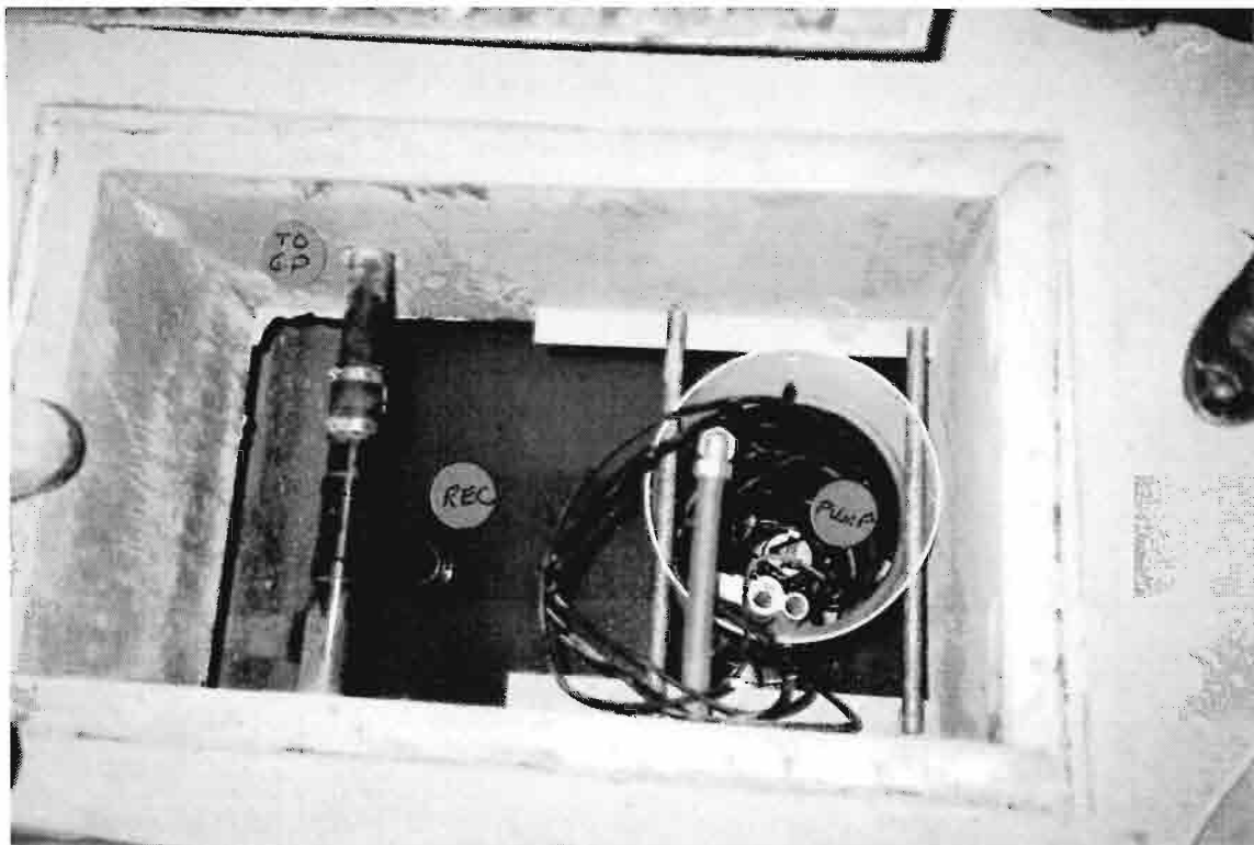
PHOTO 1-20 BIOFILTER RECIRCULATION TANK
