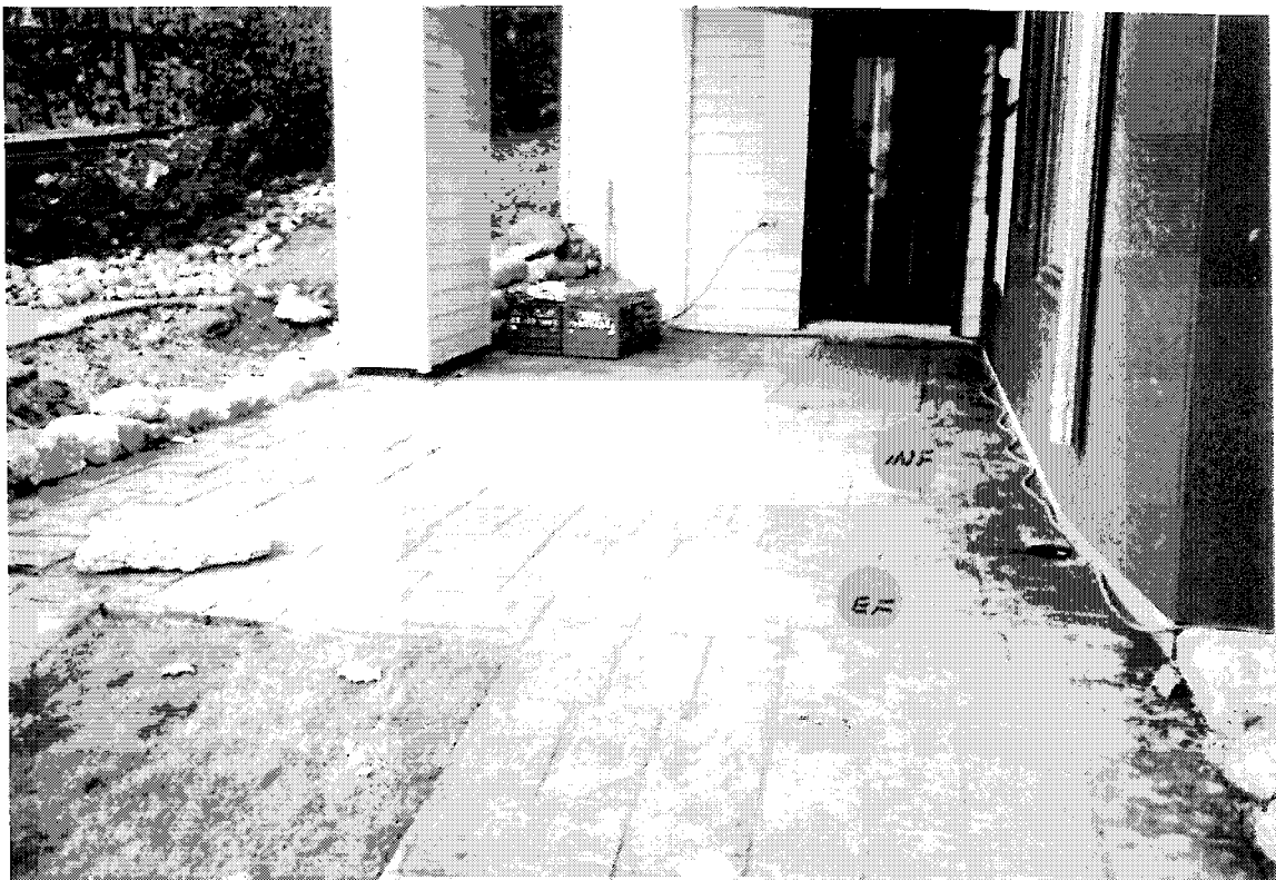
PHOTO 1-16 SEPTIC TANK UNDER CARPORT
