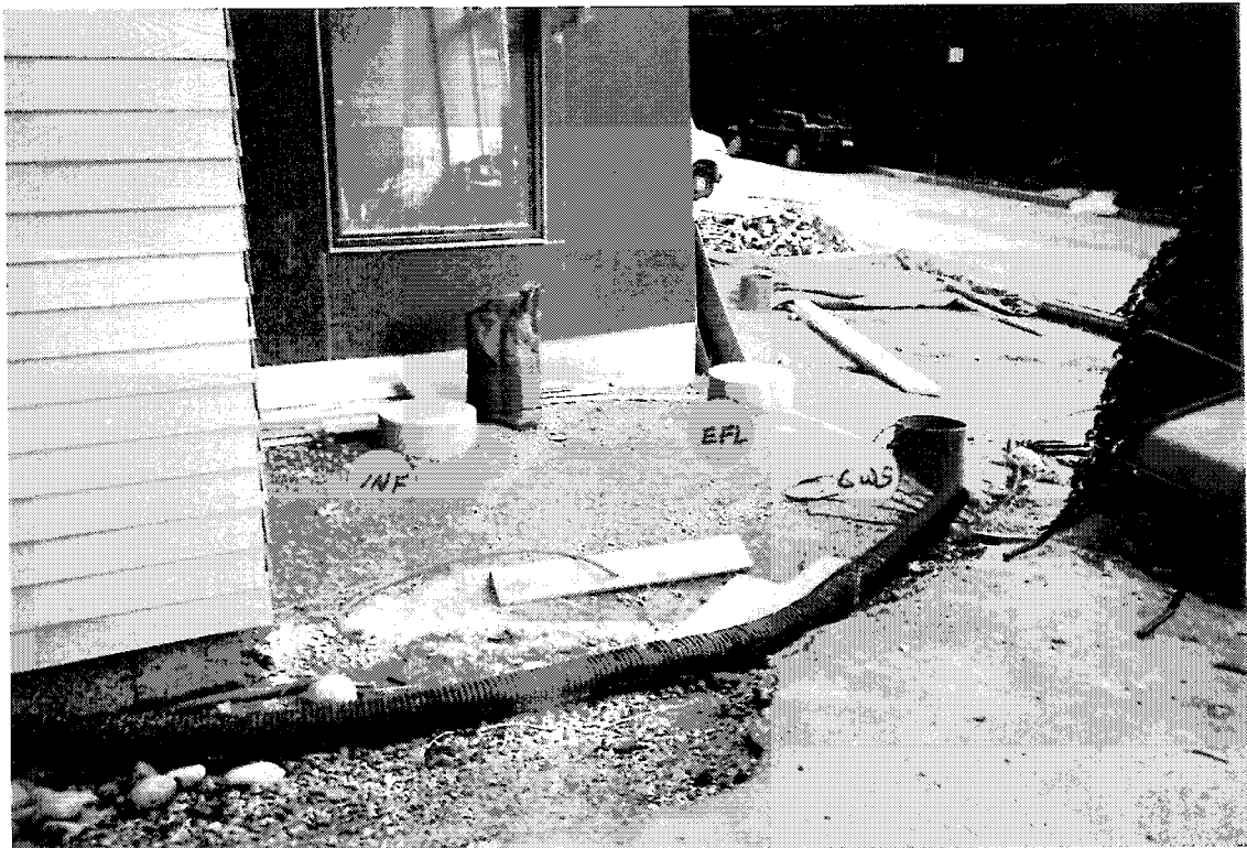
PHOTO 1-6 GROUND WATER COLLECTION SUMP
