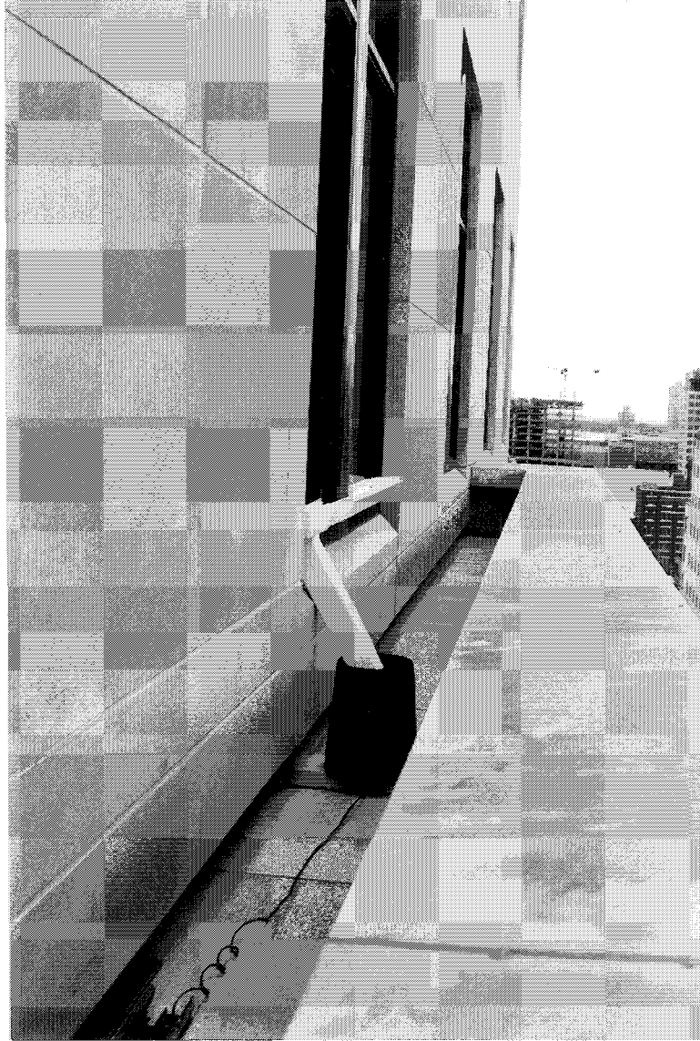
Figure (3): Arrangement of Rain Water Collection Trough and Rain Gauges
