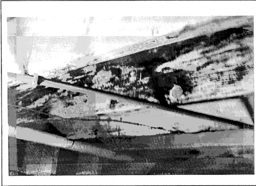
Figure 12: Mould Growth on Joists in Crawl Space
