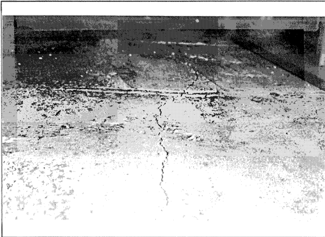
Figure 9: Cracks in concrete skin coat.
