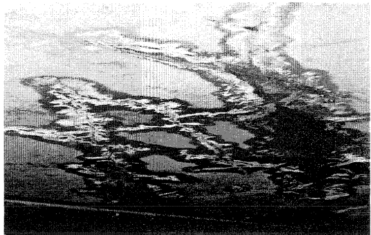
Figure 1-3 Leaching and Efflorescence
