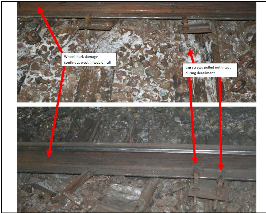
Photo 1. Track damage on high rail
