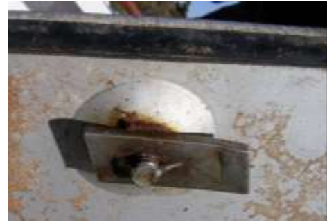
Photo 10. Underside of Lady Jacqueline hatch cover showing typical dog used for securing, found in open position
