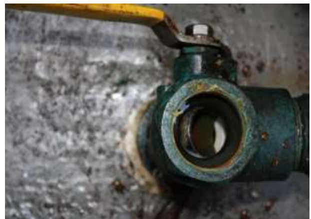
Photo 4. Three-way valve partially open to the sea
