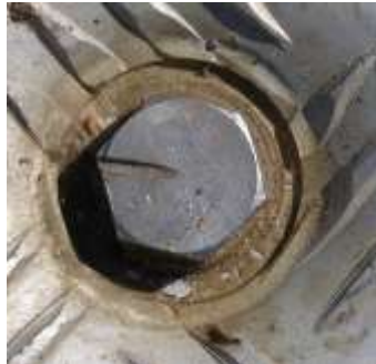
Photo 9. Typical hexagonal bolt on hatch cover
