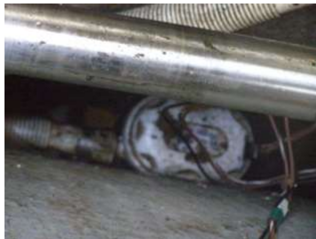
Photo 5. Position of electrical pump underneath the propulsion shaft
