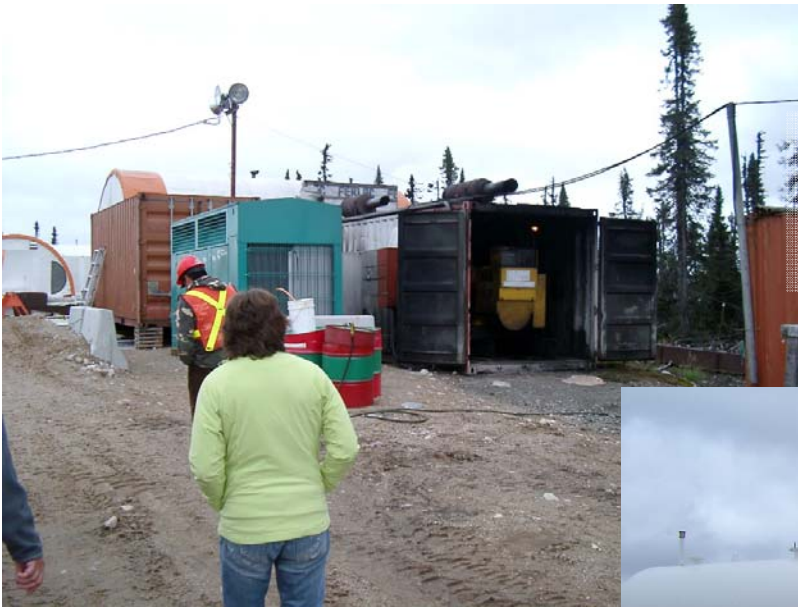
Generator with 300 kilowatts of power for the camp
