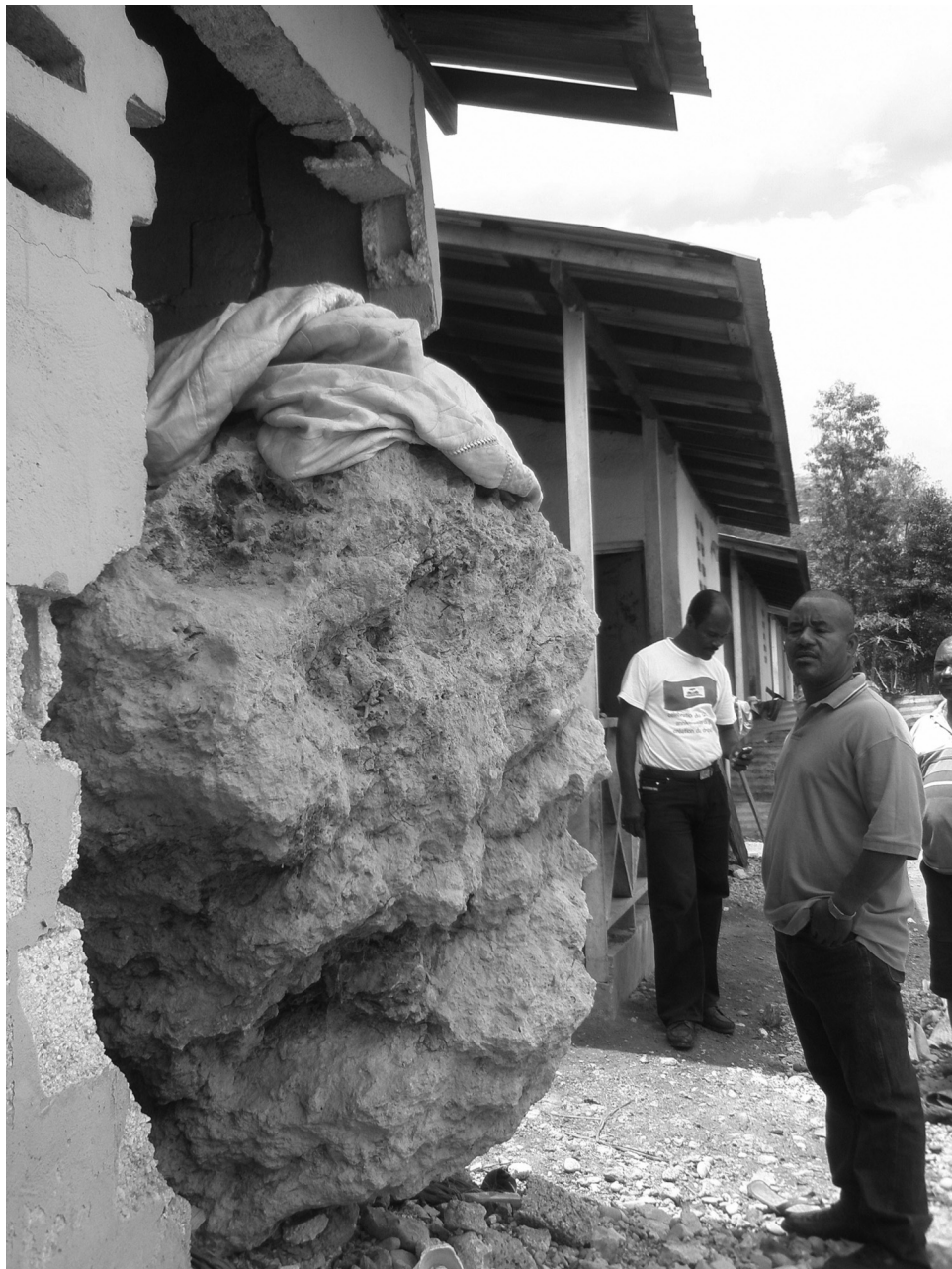
This house, built with assistance from an international NGO, was constructed in an area subject to rock slides.
