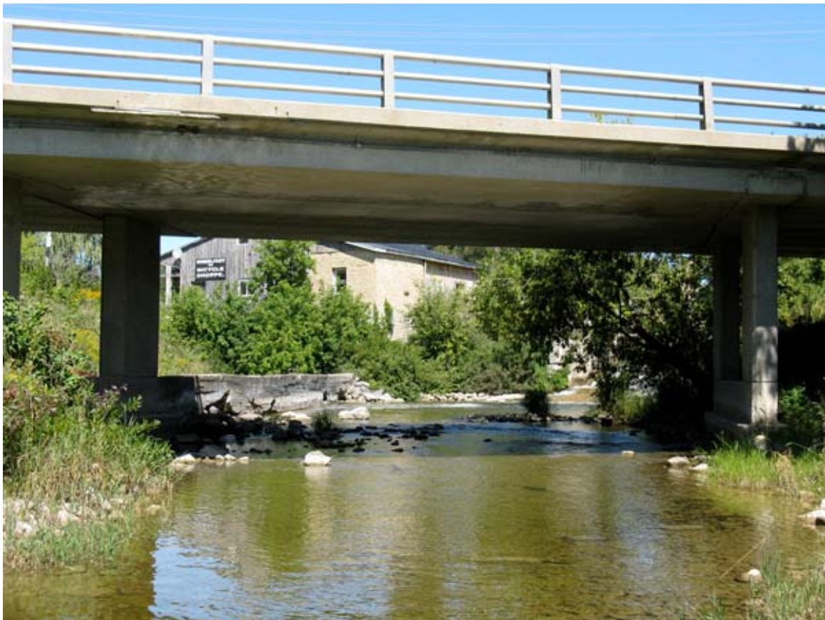
Figure 9. Looking upstream along the main river channel toward the dam at the Hungerford's Crawling Water Beetle site on the North Saugeen River, Ontario in August 2008. NE from 44.305°N 81.076°W. Photo by C.D. Jones.
