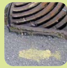
Marked storm drain Photo : © Shelley Schnurr
