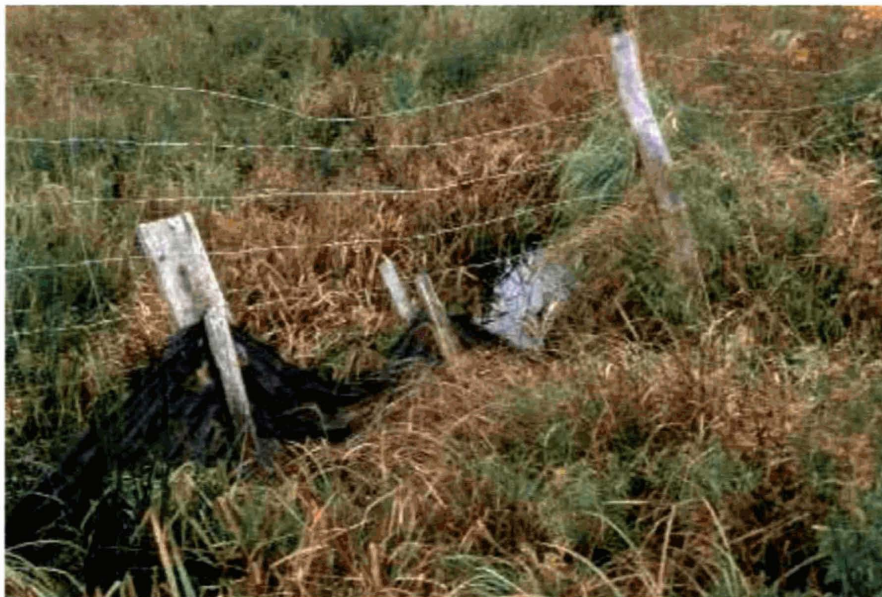
Figure 6: Improperly installed silt fence.
