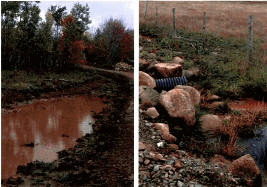
Figure 12: Private forest road and culvert construction with resulting siltation.
