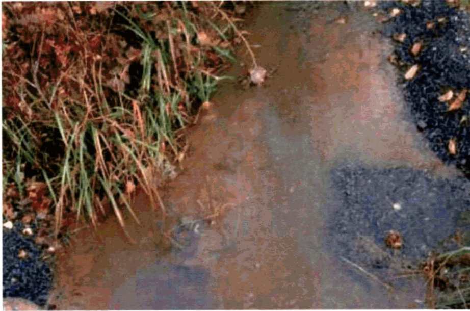
Figure 15: Streambed covered by road gravel.
