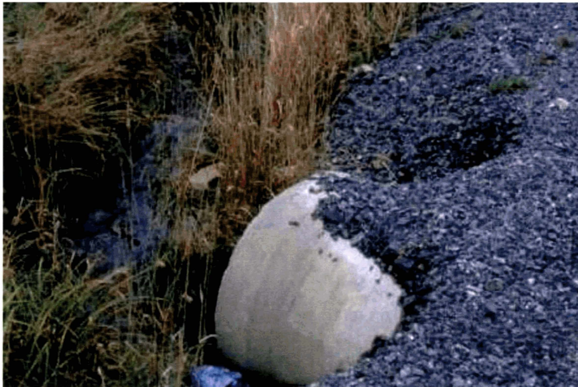
Figure 14: Inappropriately installed culvert resulting in road failure.
