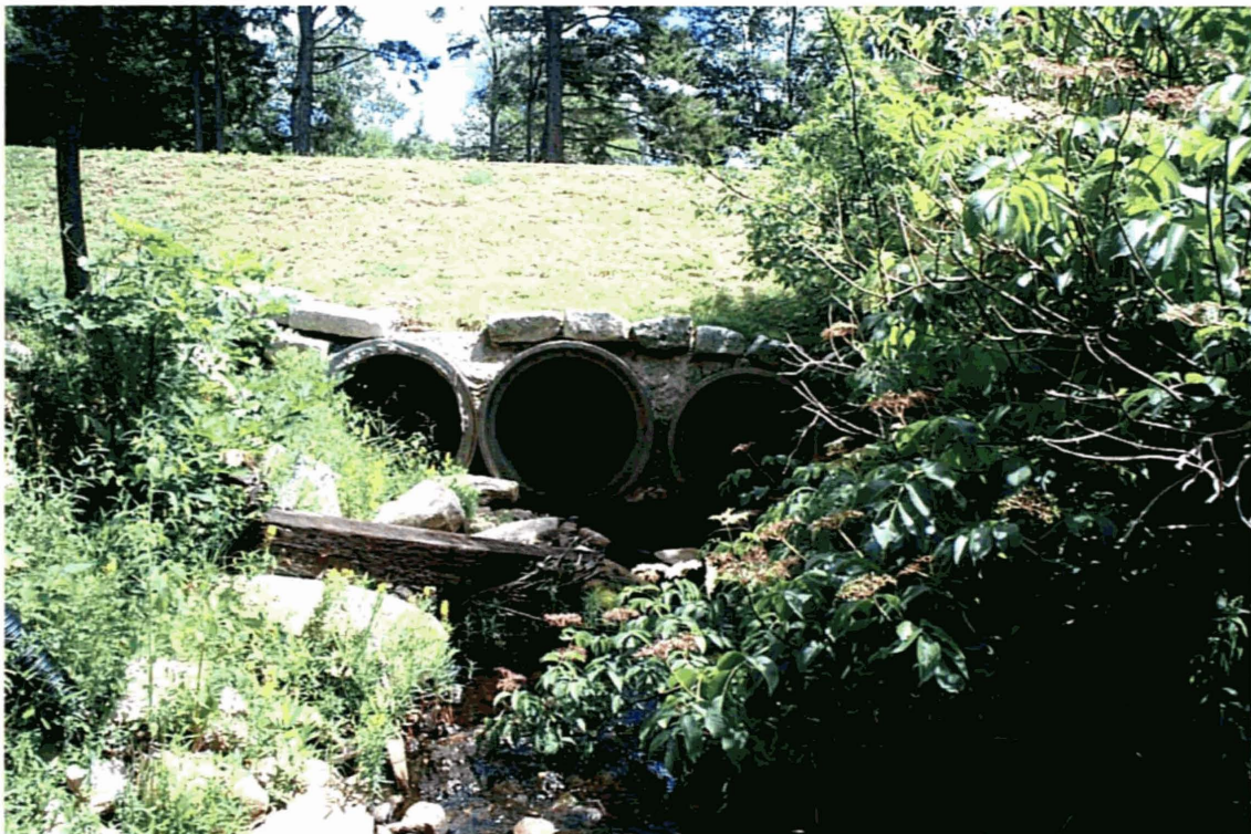
Figure 10: Culverts not installed as indicated in original notifications.
