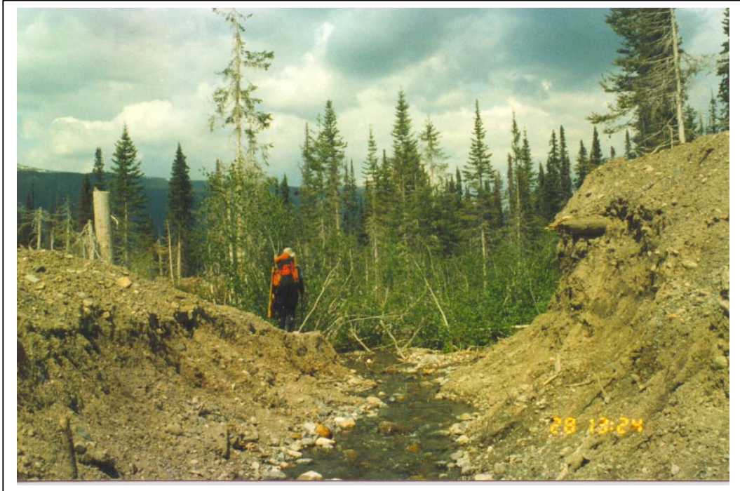
Figure 9: View of the steep, unstable cutbanks left after the removal of the culvert. This site is located approximately 200m upstream of the B5 monitoring site.
