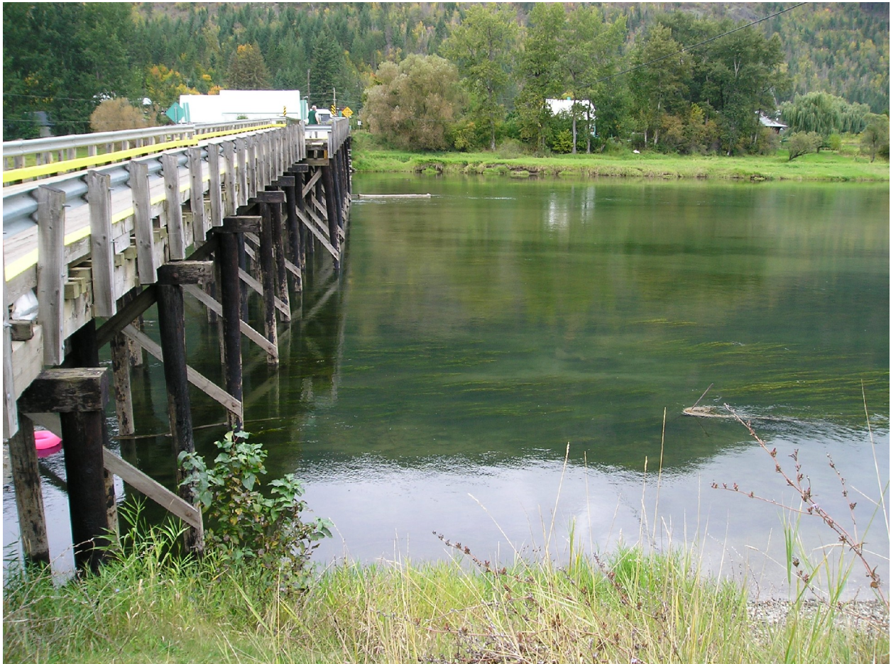
Figure 18. Bridge crossing from Riverside Drive (right bank) over the lower Shuswap River to Mara (left bank). The second of four potential DIDSON sites between Mara Lake and Enderby. Photo taken from right bank on 23 Sept 2004.
