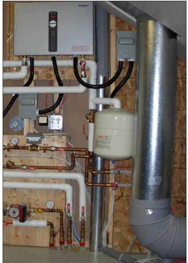
Figure 1 Tankless Water Heater installed at Avalon Discovery 3
