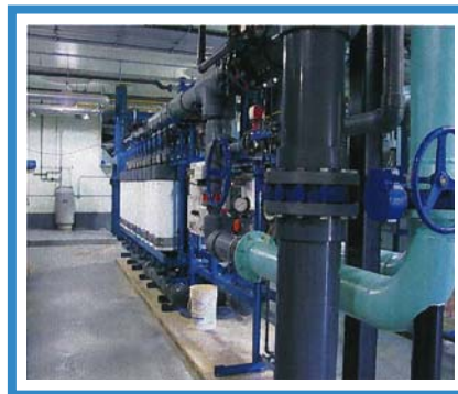
Above: The Lac La Ronge Regional Water System Water Treatment Plant
