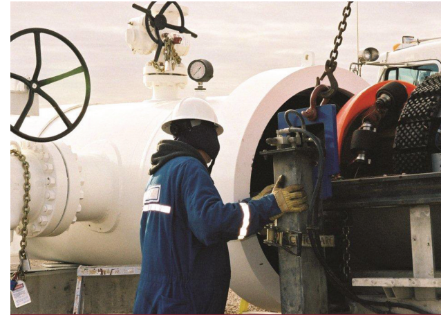
In-line inspection tool - Photo courtesy of TransCanada
