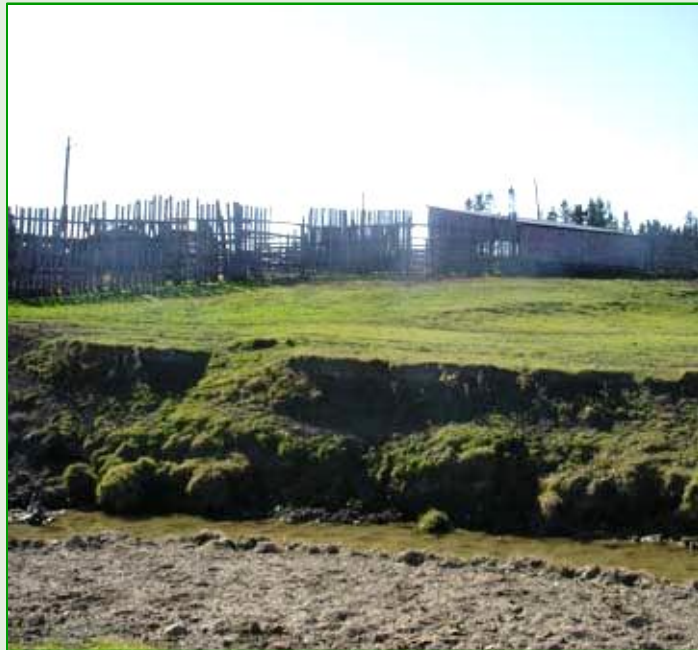
Unstable and eroded banks of the Renicker Creek resulting from livestock activity adjacent to the former confinement facility
