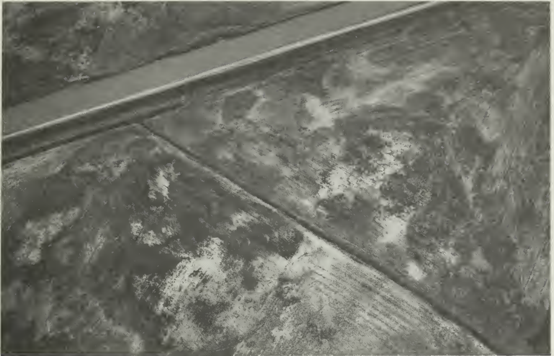
Fig. 6. Damage caused by seepage from canal.
