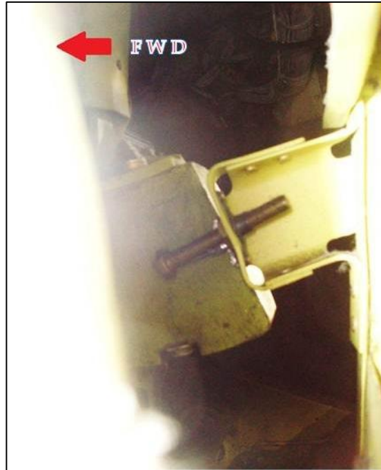
Photo 2. Bob-weight aligned with damaged area
