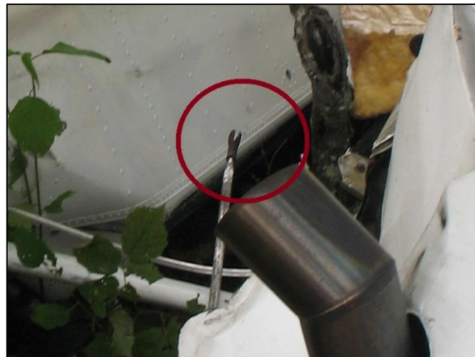
Photo 2. Bracing wire with clevis pin missing
