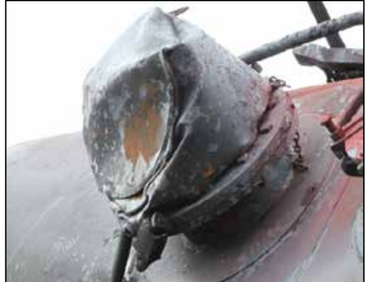
Photo 22. Hinged housing for tank car fittings
