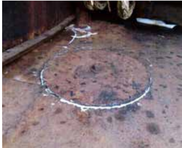
Photo 3. Silicon sealant on 1 of the 26 hatch covers
