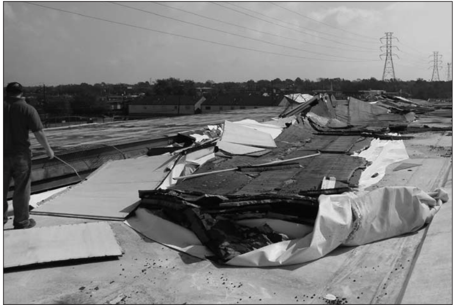
Commercial roof cladding failure as a result of high winds
