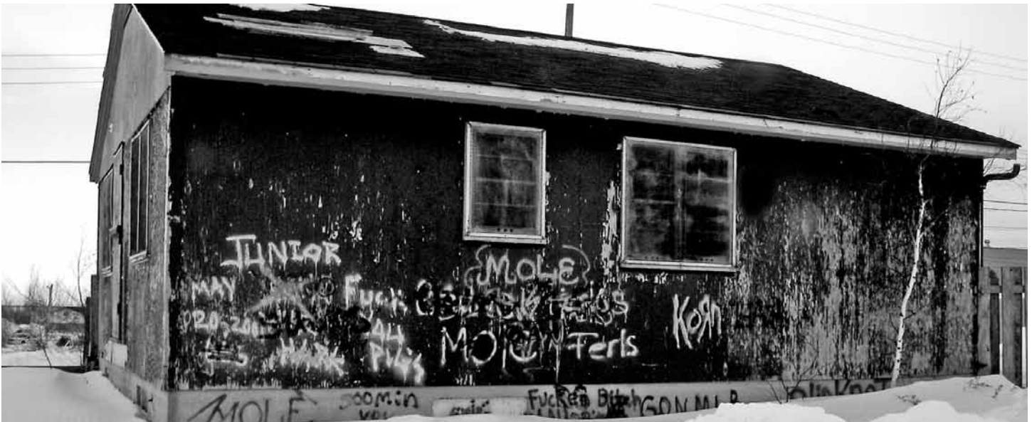
Graffiti and property damage are a widespread issue in northern Manitoba.
