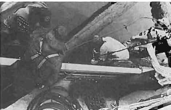
Plate 1-2. Pond No. 1 construction. The seawall corner of the pond is being triangularized to strengthen the pond frame.
