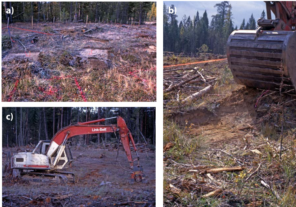
Figure 4. Establishment of satellite plots a) outlined in paint and then treated (as applicable) with b) excavation and c) compaction (excavator fitted with vibrating plate).
