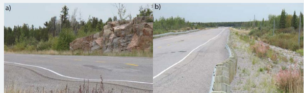
FIGURE 4: Photographs of Highway 3 indicating a) differential subsidence of the road surface and b) guardrail displacement caused by rotational down slope movement of the highway embankment side slope (Source: Stevens et al., 2012).
