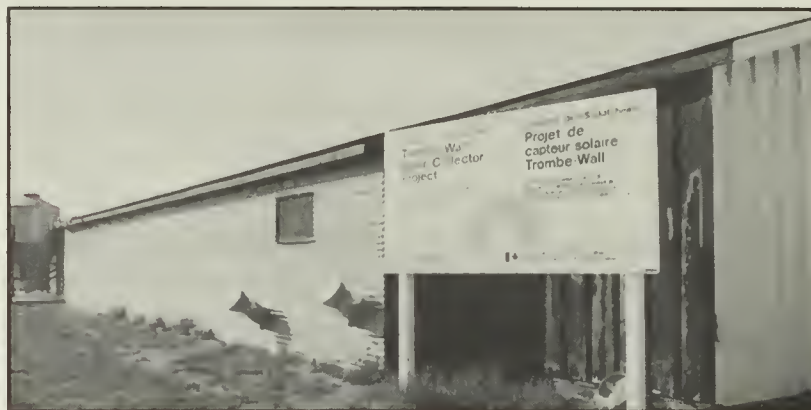
Fig. 8.2 A Solar Wall For Preheating Ventilation Air In a Swine Barn
