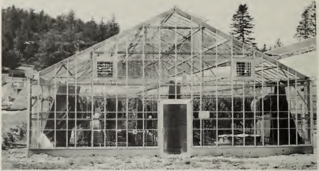
Fig. 6. An even-span gable greenhouse with the sidewall ventilator opened first, followed by the leeward ridge ventilator.
