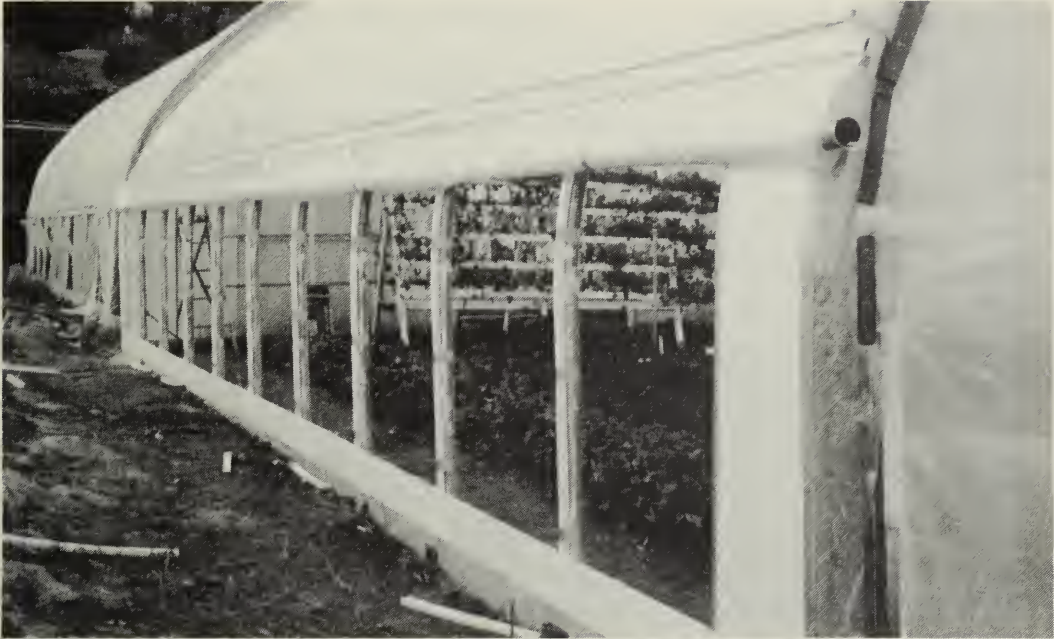
Fig. 8. A polyethylene sidewall ventilator rolled up on shaft.
