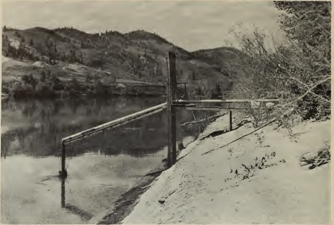
Figure 3. River intake, which can be moved up and down as the water level changes.
