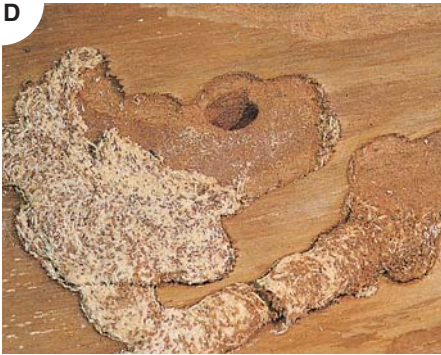
T. castaneum gallery filled with brown, granular frass. Note exit hole (5 mm wide).
