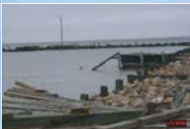
Wharf damage at Escuminac
