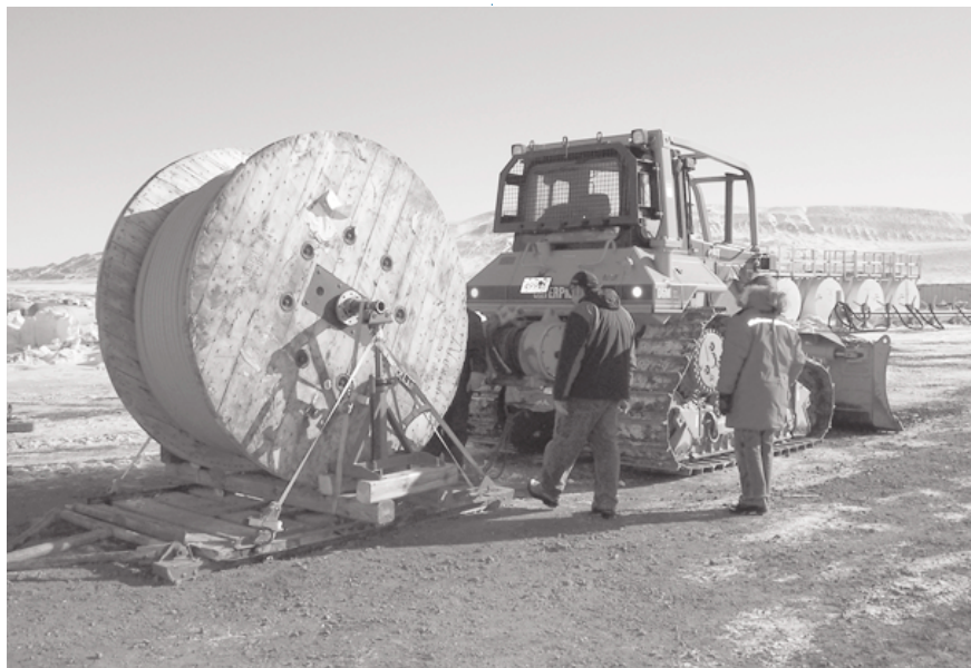
Figure 3 Laying the power cable for the new SAFIRE site which is 2km from the nearest supply. The 'dozer drags the sled with the reel (weighing 6,500 kg) across the frozen ground paying out the orange power cable behind. Photo: Jim Drummond.
