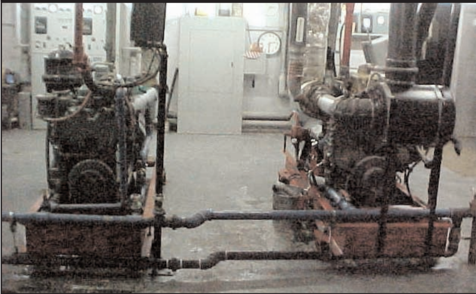
Original Generator System—Still in Operation
