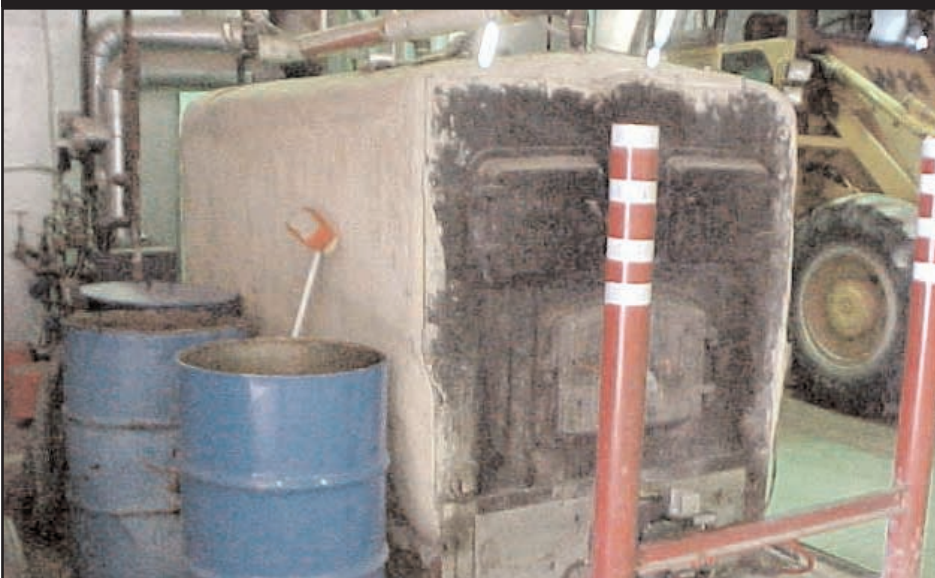
Heat Exchanger (cast iron, biomass Converter furnace)
