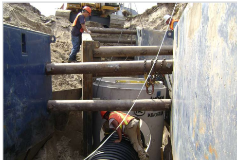
Contractors installing a 900mm storm pipe during the private military quarters (PMQ) Municipal Works Upgrade Project, which took place this summer and fall.
