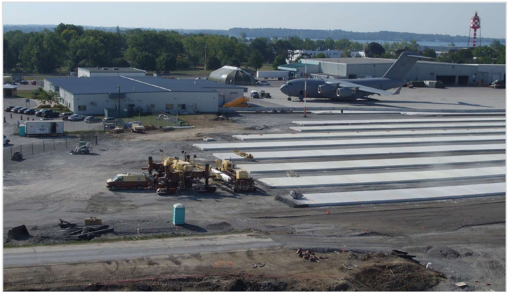
The first phase of a $90-million apron replacement program — a $15-million project to replace 40,000 square meters — was completed in November.
