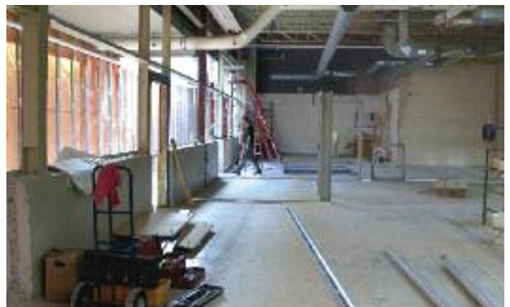
Work underway in the Vulcan Building to accommodate shops relocated from the van Steenburg Building
